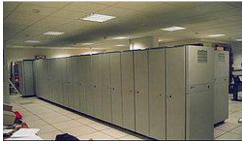
Nortel sl-100 Telephone Switch In Glover
